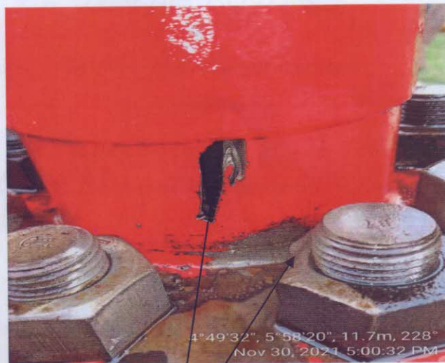
SPILL POINT (LONGITUDINAL FRACTURE OF TH CHOKE BEAN ADATER AND ABRASIVE WEAR OF THE OUTER SURFACE OF CHOKE CORNER)
